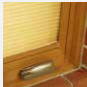
DOES NOT PROTRUDE
